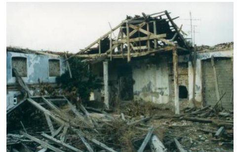
The state of the Beth El synagogue in Komotini is surveyed by the writer in 1993, a year prior to its demolition
